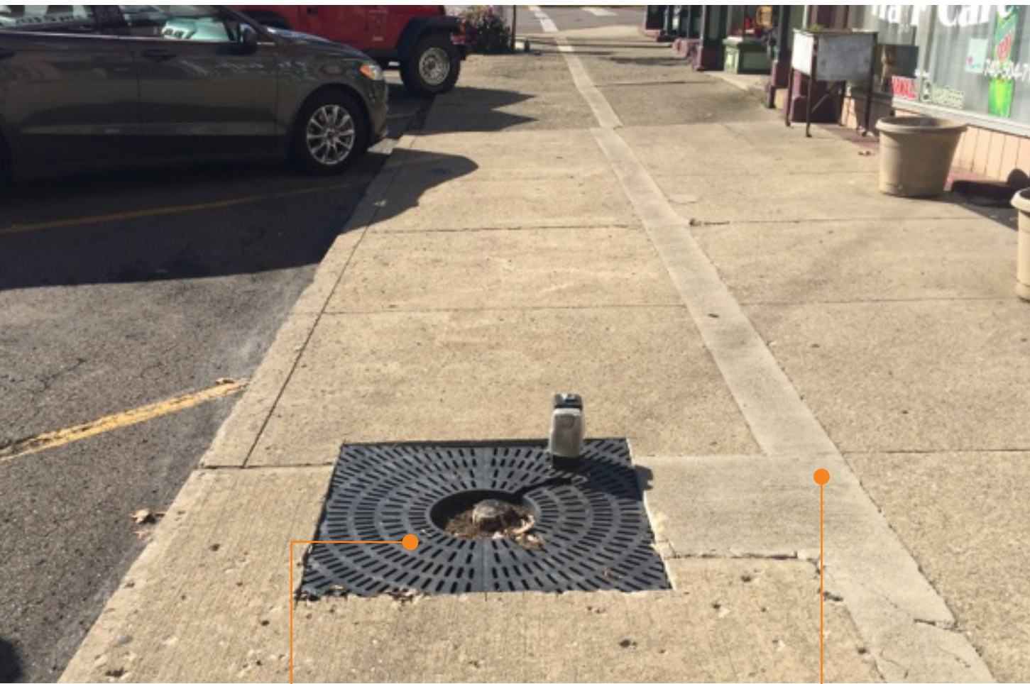
Missing and non-uniform street trees and grates
