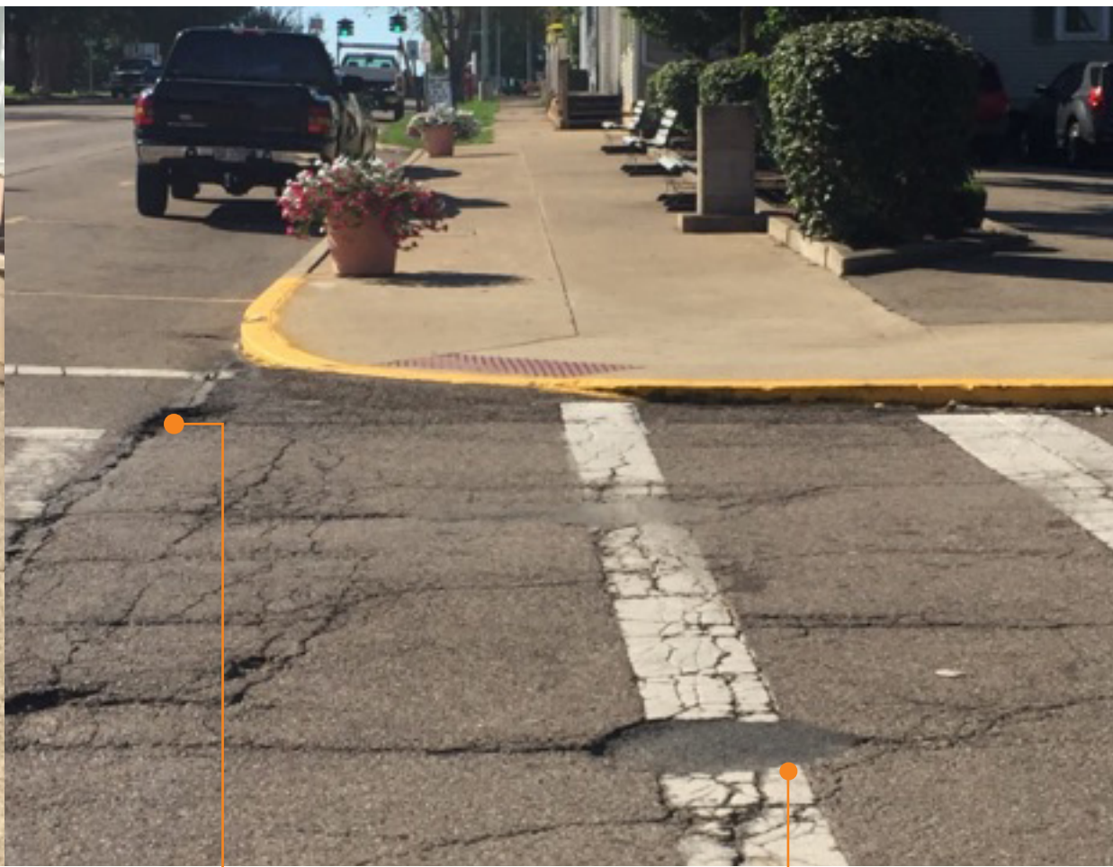
Presence of potholes and large cracks
